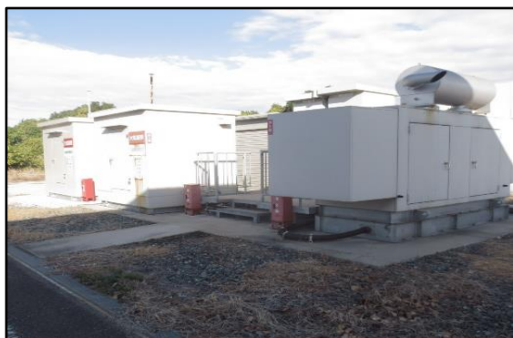
Elevated installation of an emergency generator
