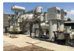
ITS power receiving and transforming facility
