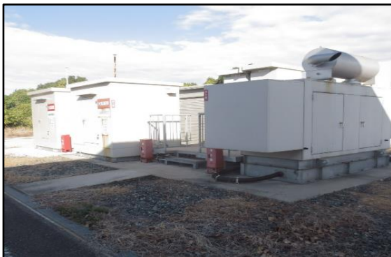
Elevated installation of an emergency generator
