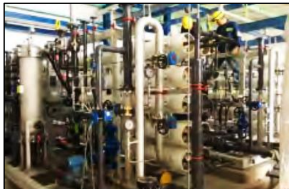
Reuse of plant wastewater using water treatment membranes
