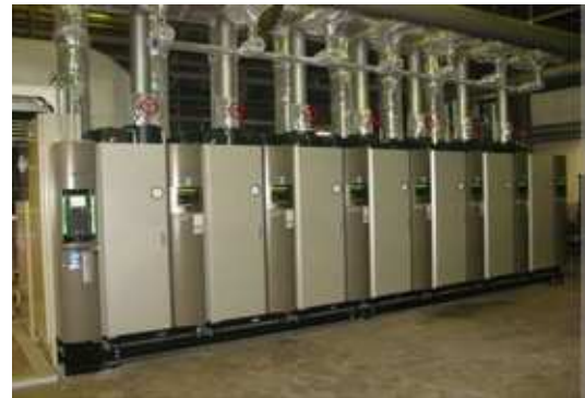
Natural gas boilers at the Aichi Plant
