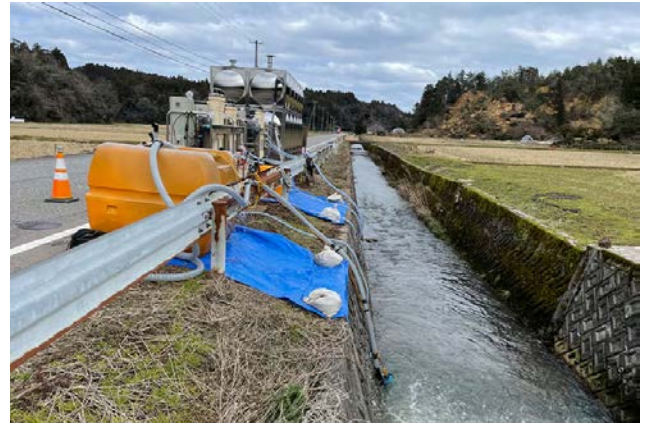
Makusesu Safety systems drawing water from a nearby river
