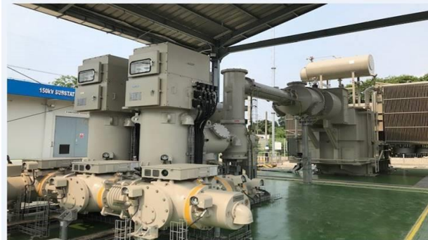
New power reception and transformation equipment enabling grid power purchasing
