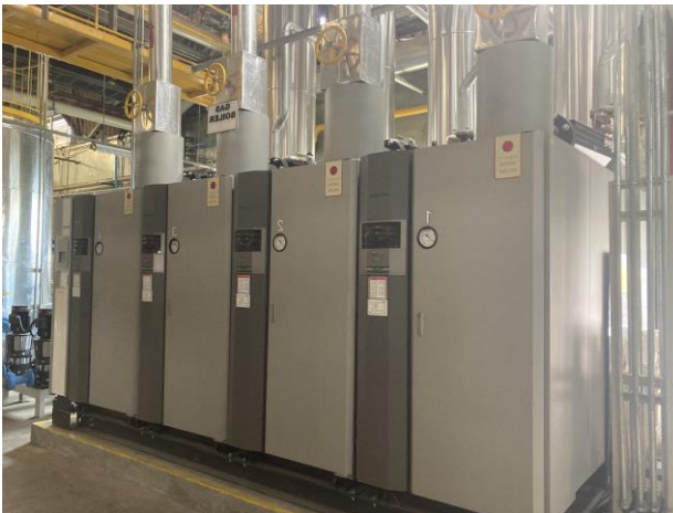
New gas boilers to enable transition to cleaner fuel
