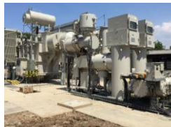
ITS power receiving and transforming equipment
