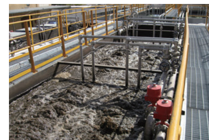
Toray MBRが設置された下廃水タンク Wastewater Tank in which Toray MBR are installed
